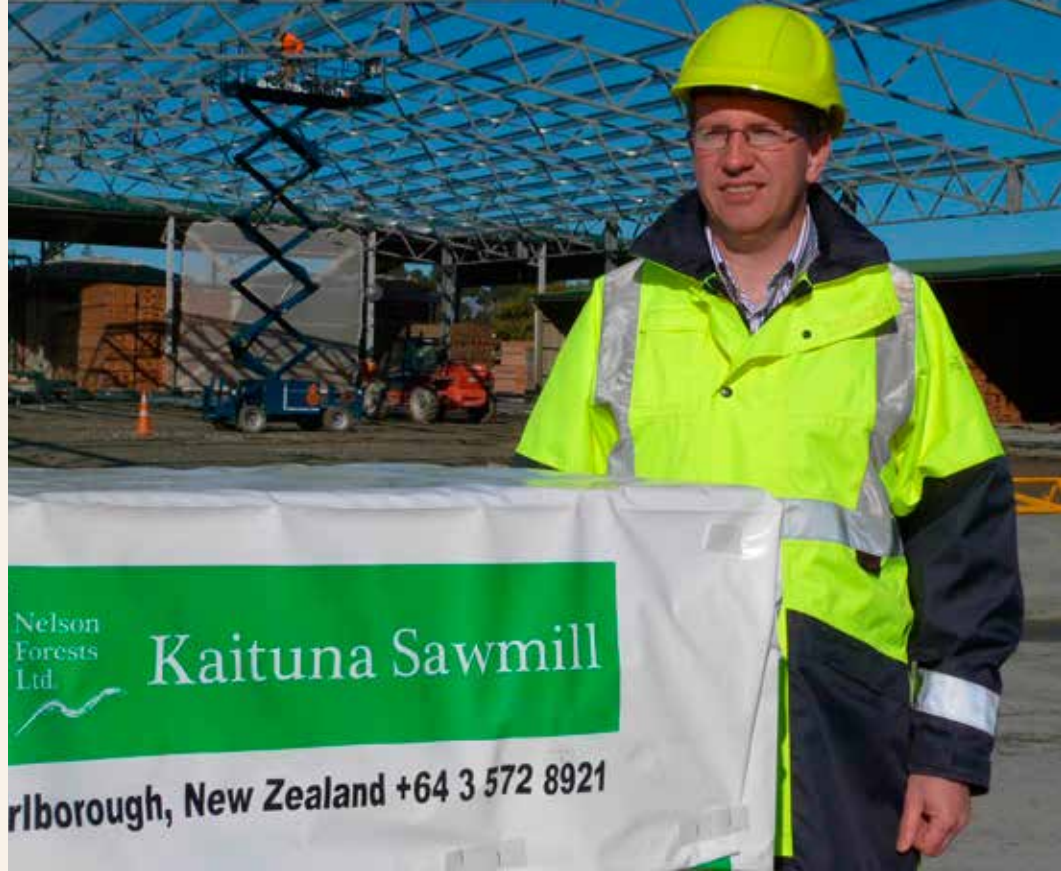
Kaituna Sawmill's Site Manager Darrell O'Brien with the new high span dry storage building that is currently under construction
